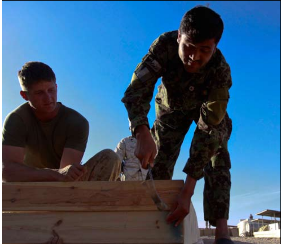
An Afghan National Army soldier puts the final touches on the foundation of a building, which will be used for a combat operations center aboard Camp Garm-sher, Afghanistan, Dec. 10.
